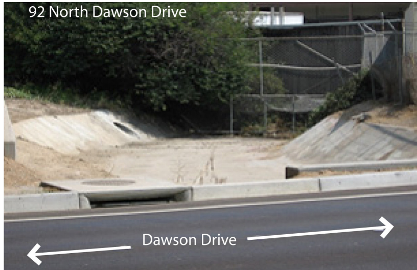
Another site known to city staff to have a history of flooding and an unusual drainage system is the rental yard at 92 North Dawson Drive.
