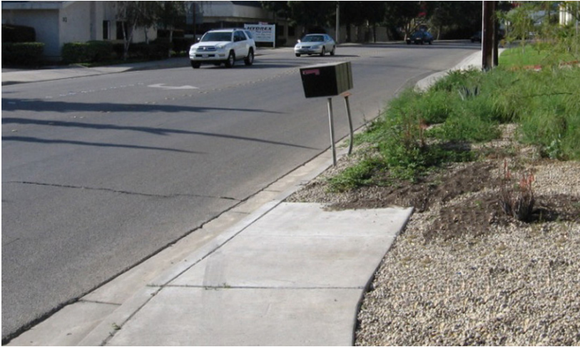
Existing lack of sidewalk continuity on South Dawson Drive.
